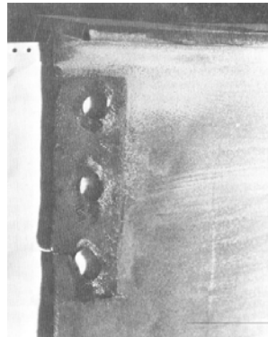
Figure 6.137 : Fractured beam web of a double angle bolted connection (Birkemoe et al. 1978)
