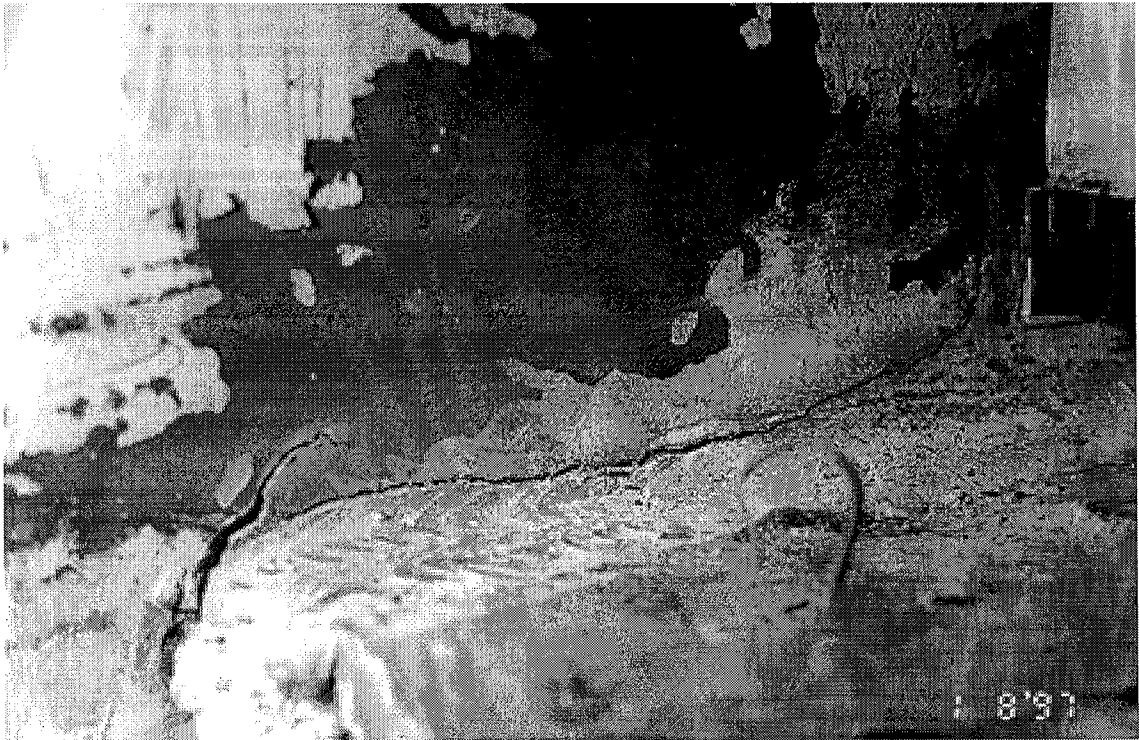
Figure 3.11: Pull Out-Type Failure of Column Flange (West Girder of Specimen 2)
