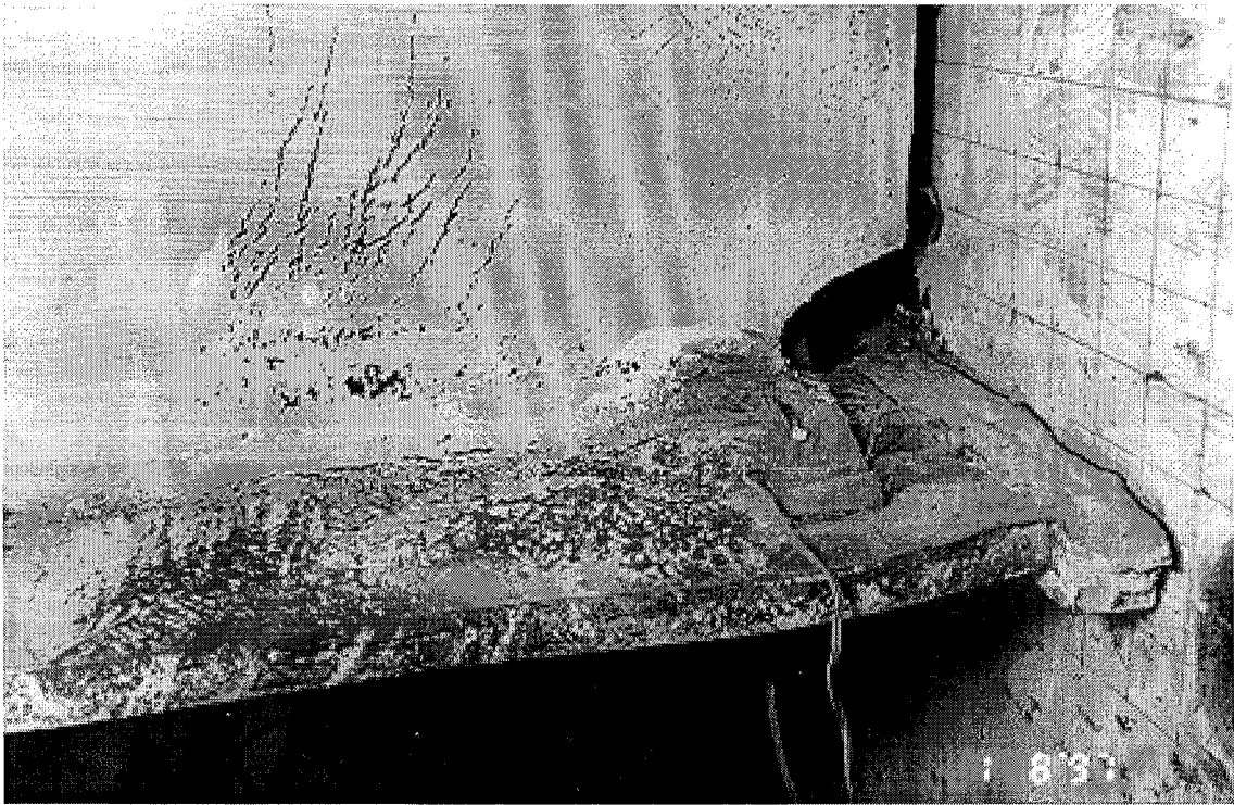
Figure 5.60: Fracture of Bottom CJP Weld (East Girder of Specimen 2)
