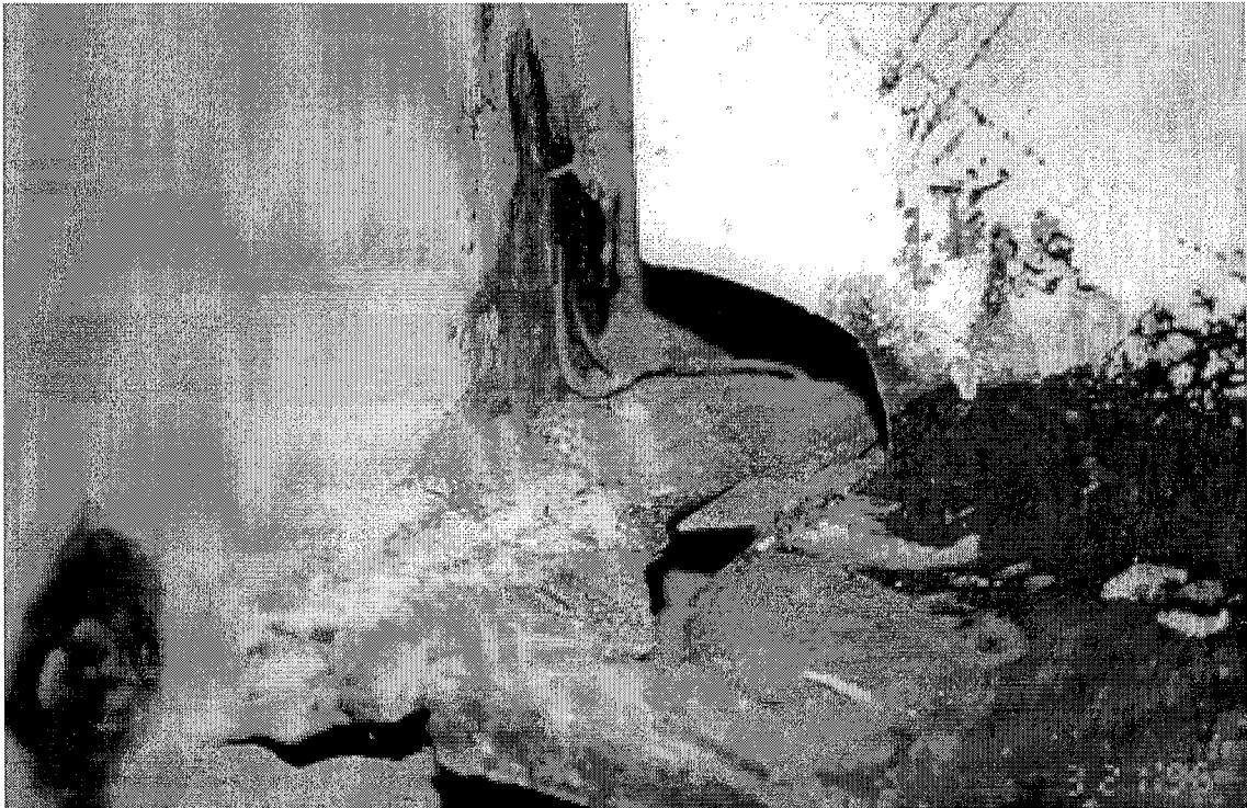
Figure 3.17: Rupture of Girder Bottom Flange (West Girder of Specimen 3)
