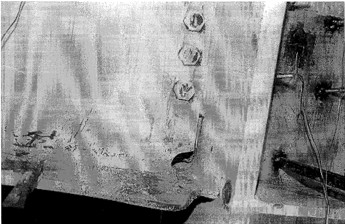
Figure 5.76: Rupture of Bottom Girder Flange (East Girder of Specimen 3)
