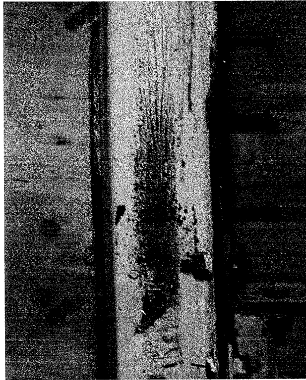
Fig. 4.4.3 Bottom Portion of the North Column in the Second Story after Testing
